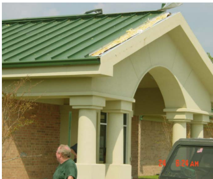
Figure 5: Damage to the roof, Gulfport, Mississippi, District Office
