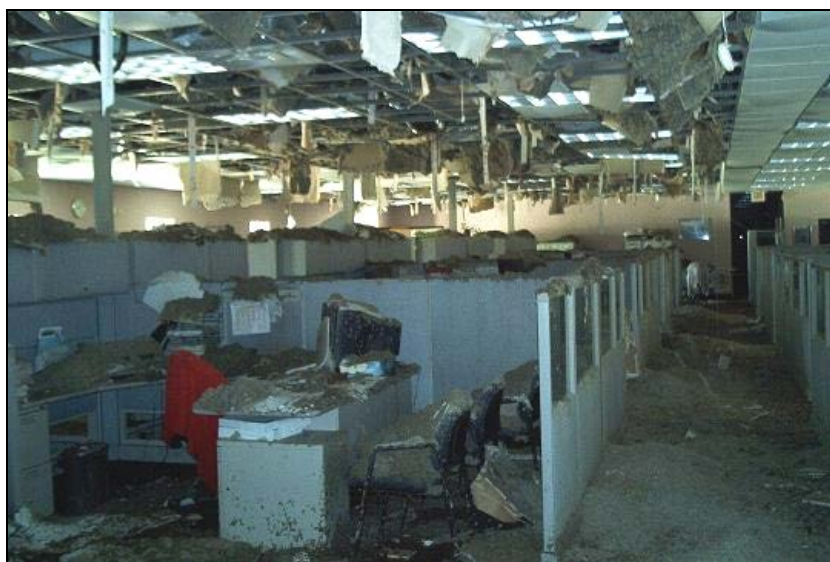
Figure 1: Inside the Kenner, Louisiana, District Office
